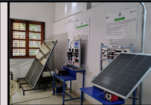
RENEWABLE ENERGY LAB
